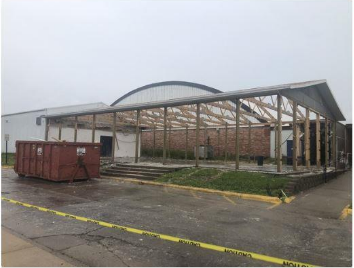
The old weight room / training room being demolished to make room for new classrooms! Awesome improvements underway !
